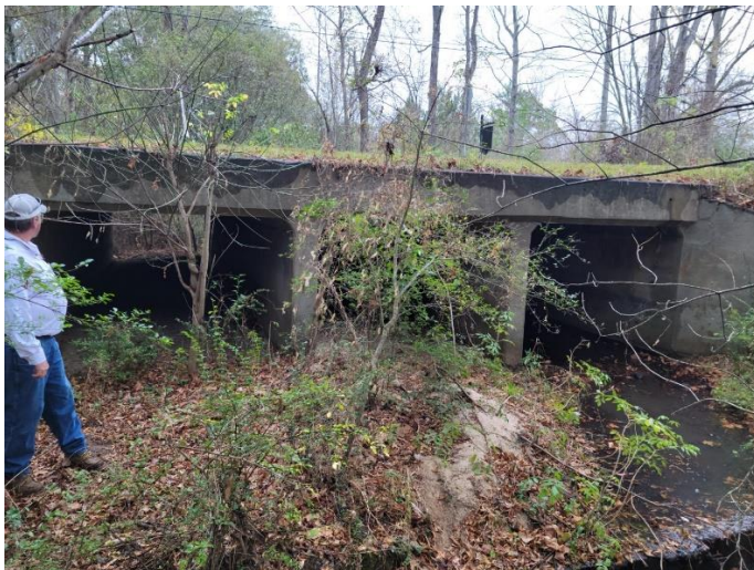
Dried Indian Creek on E. Soule Street - 9'x6' Triple Boxed Concrete Culvert that is approximately 11 year's old. The County does not feel it would support the weight for commercial/industrial development that is contemplated near this site.
